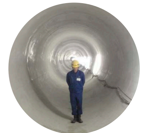
中村西部雨水調整池 Nakamuraiseibu Stormwater Storage Facility
